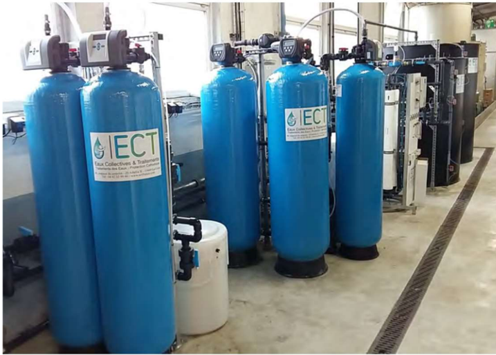
Reverse osmosis line for a washing tunnel including a de-manganisation station, an iron removal station and an ion exchange resin softening station.
